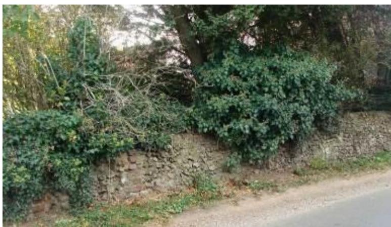
Picture 15: Wall at Gravesend Farm that would benefit from repair work and removal of ivy
